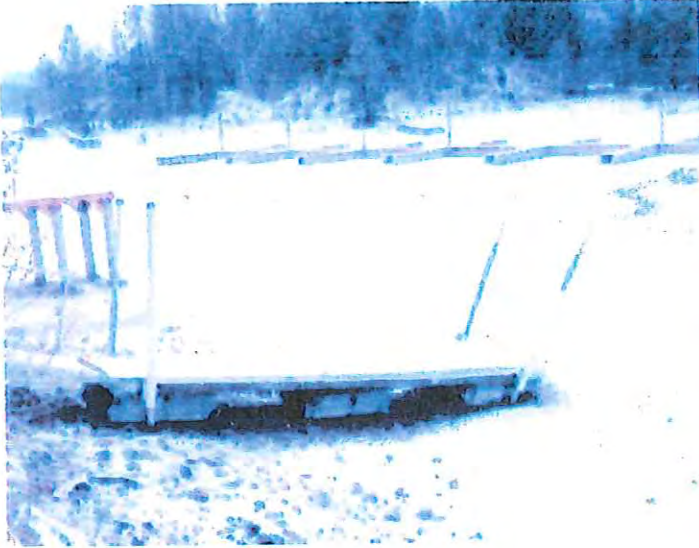
Dock One Broken
