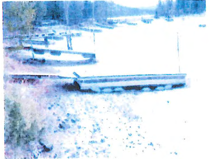
Dock Nineteen Broken
