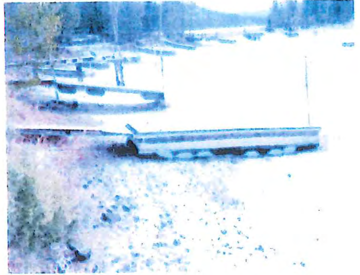
Dock Nineteen Broken
