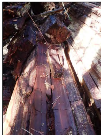
Figure 23. Extensive brown cubical butt rot from Schweinitzii root and butt rot.
