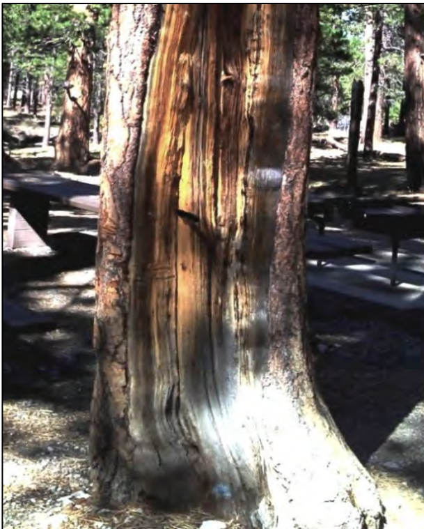
Figure 10. This Jeffrey pine had a large basal wound affecting slightly less than 30% of the stem's circumference and 4-6 in. deep, lengthwise cracks in the exposed wood.
