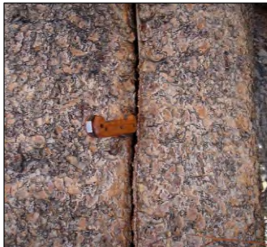
Figure 77. The sides of this deep crack move independently past each other, indicating high failure potential (FP 4).
