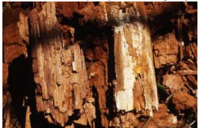
Figure 6. Brown cubical decay.
